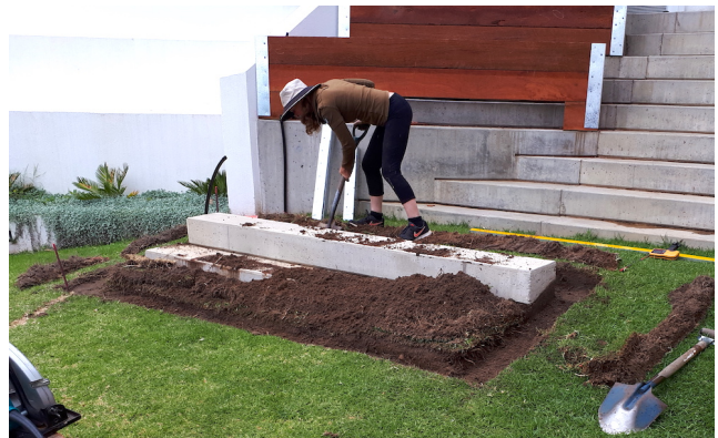
Digging out the soil, ready for placing the 4 panels of the garden bed.
