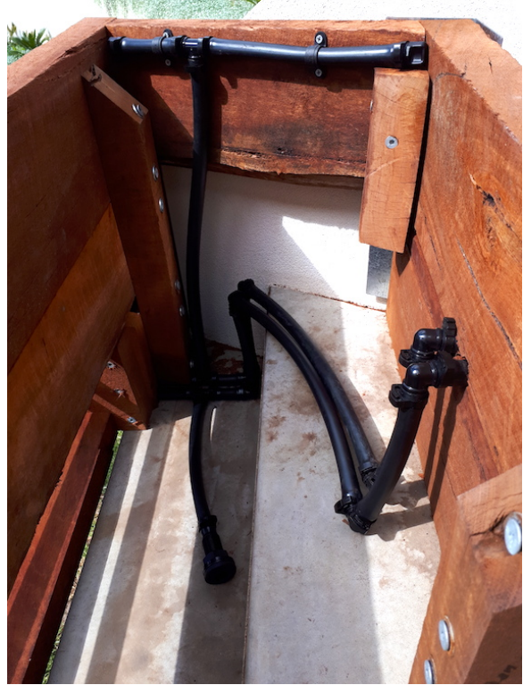
Some creative irrigation, with one pipe to let water in and one pipe to let excess water drain out
